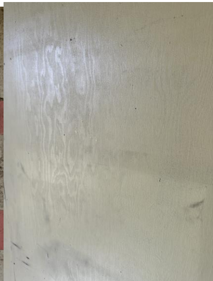
Paint on wall board
